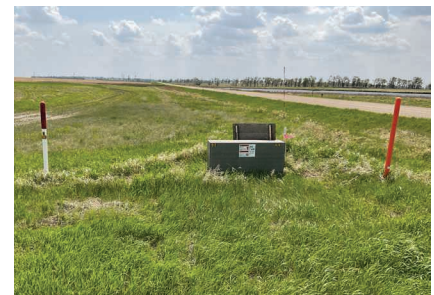
(Left) Pad-mounter transformer and meter. (Above) Three-phase cabinet.
